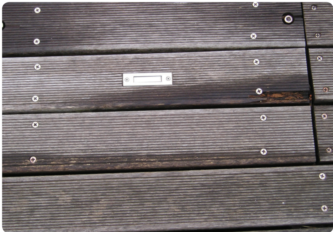
Decay in untreated sapwood on edges of decking boards.
