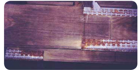
Corrosion of nail plates on deck joists after 6 years exposure near surf beach.
