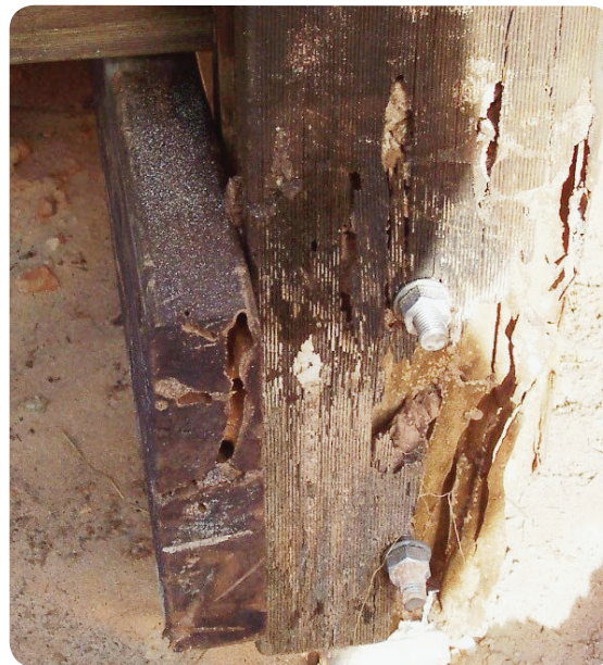
Termite damage to non-resistant timber.
