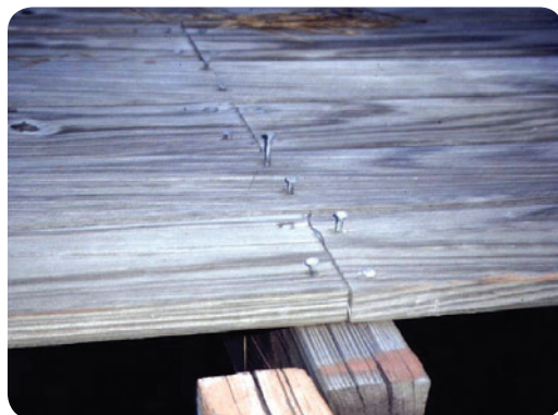
Plain shank decking nails in pine have ‘worked out’ with cyclic wetting and drying.
