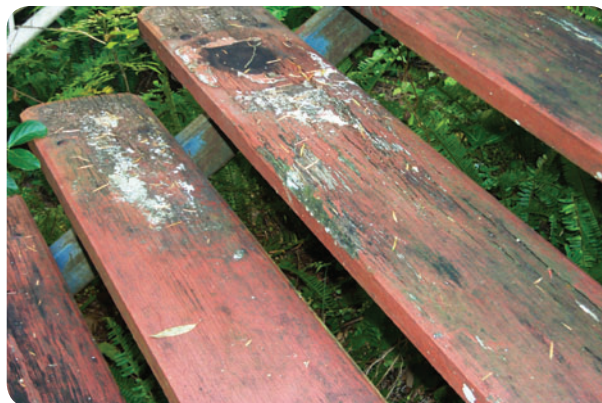
Poor maintenance of stair tread.
