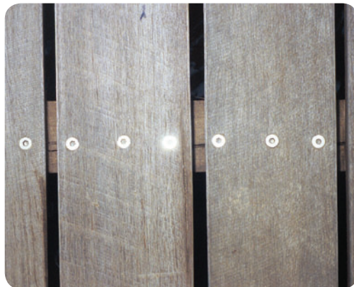
Deck screws should have been staggered to prevent splitting of joists.
