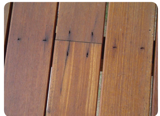
Incorrect use of non-galvanised ‘T’ head nails in decking.
