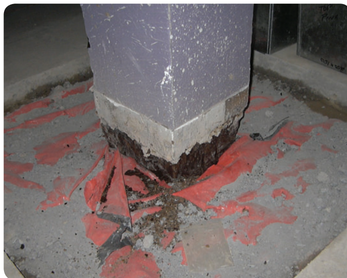
Degradation of basement column after 100 years in service in Brisbane.
