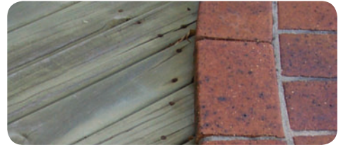
Corrosion of HDG nails close to pool edge.
