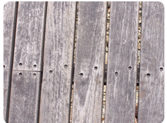
No splitting of joists where deck screws were staggered.
